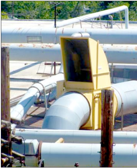
Figure 10. Abort gate in duct
