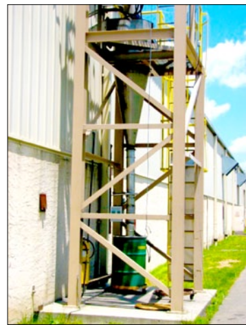
Figure 2. Cyclone dust collector
