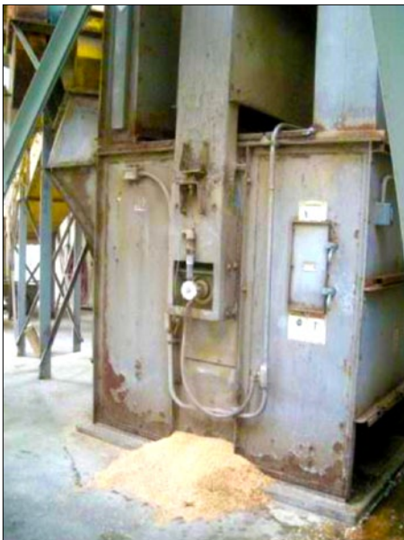
Figure 8. Sawdust spilled from equipment
