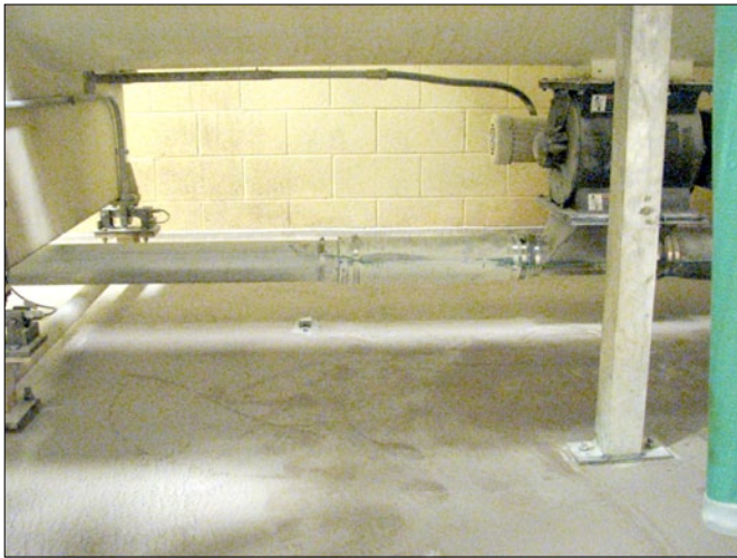
Figure 1. Conveying system piping
