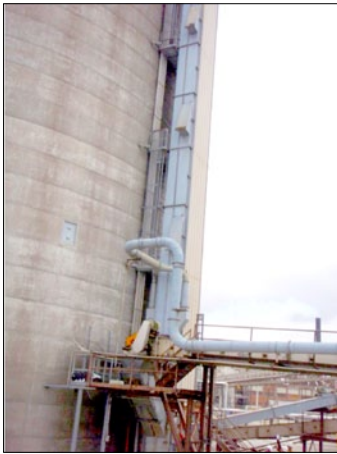
Figure 1. Bucket elevator and storage silo
