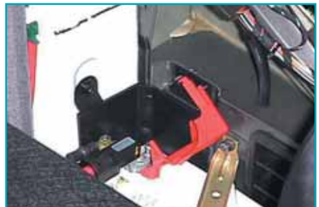
automatic disconnection system
